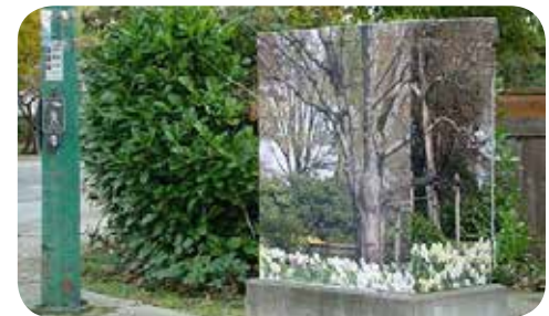
Anti-graffiti utilities box 'wrap'
