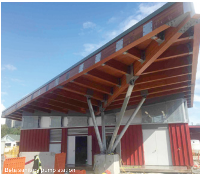
Beta sanitary pump station
