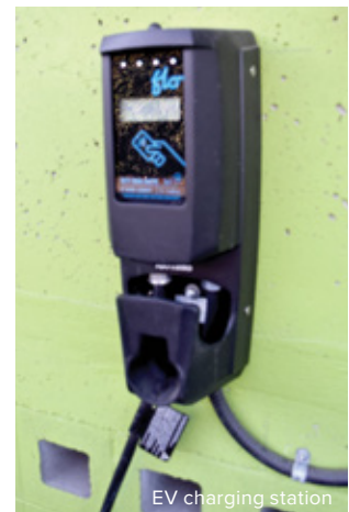
EV charging station
