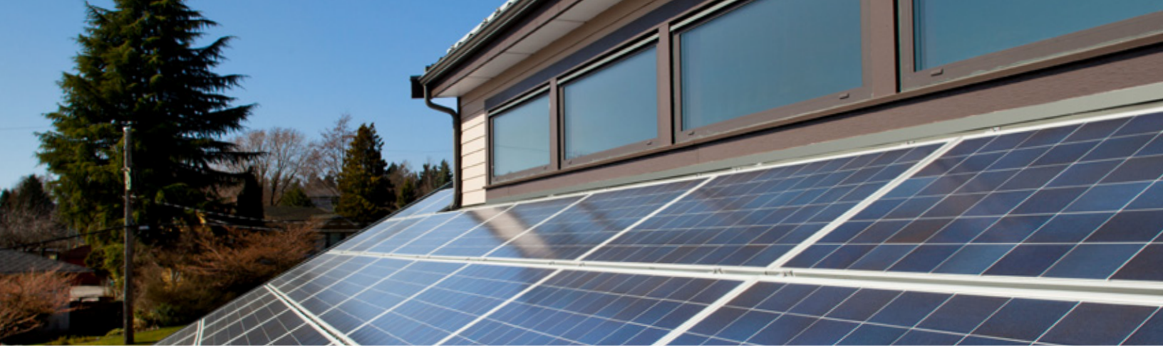
Solar Panels at Harmony House
