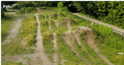
Example of jumps eroding.
